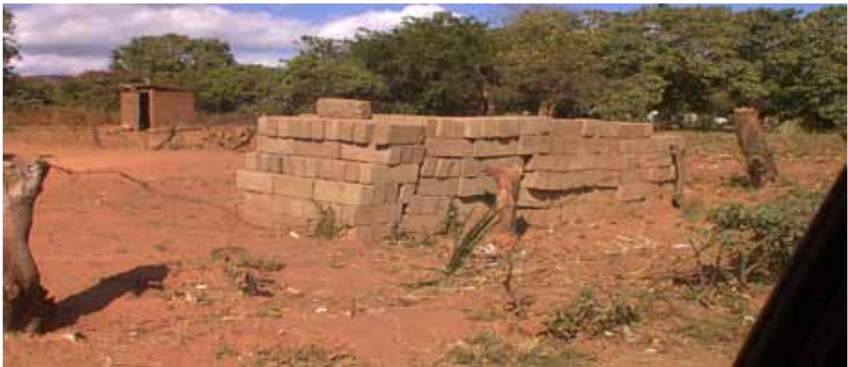
Blocks for one of the officer's in readiness to build a house at his own expense.
